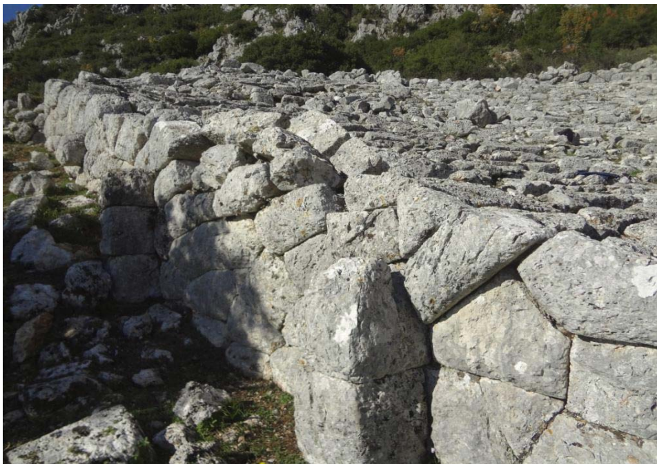
10. Detail of the western retaining wall of the auditorium after the deforestation works. (photo: Diazoma/2012)
